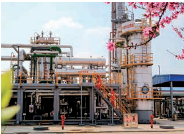
Natural gas decarbonization & recovery facilities
